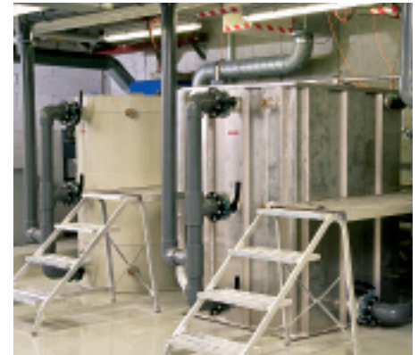
Level measurement in a water treatment plant
